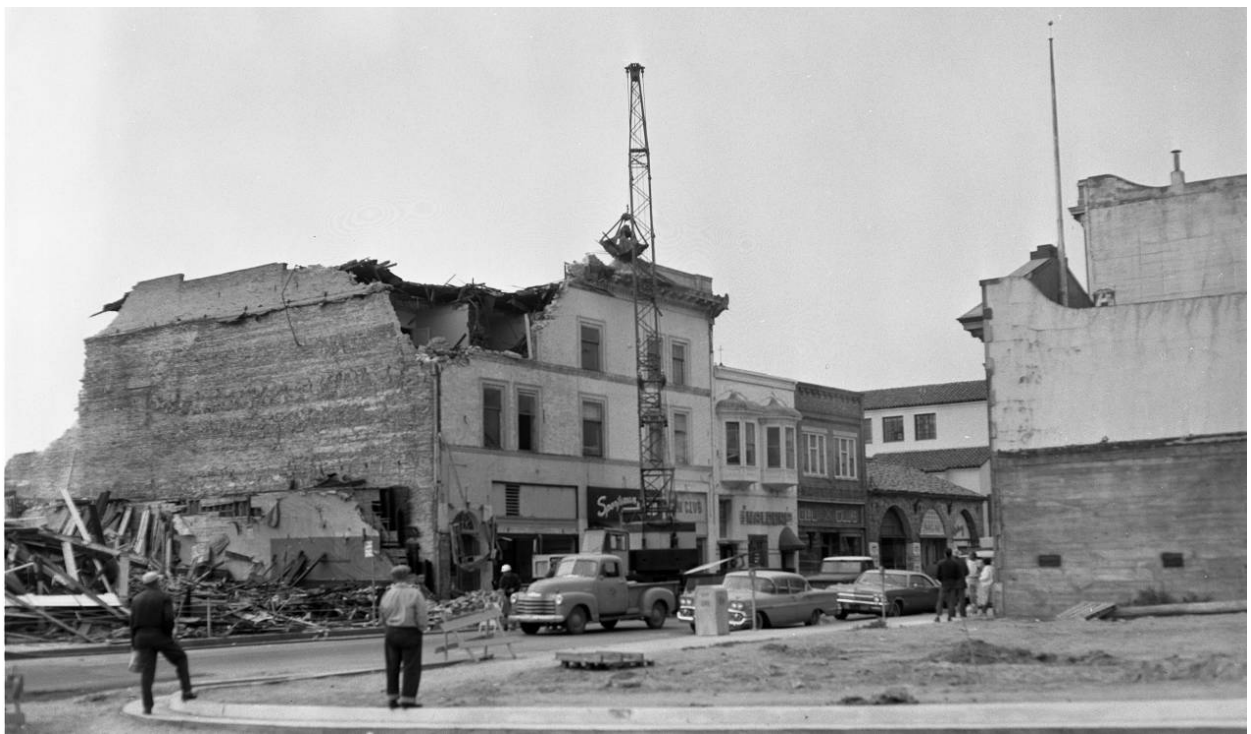
Figure 10-8. Demolition of same section, June 28, 1967 (William L. Morgan, photographer, courtesy Monterey Public Library, California History Room).
