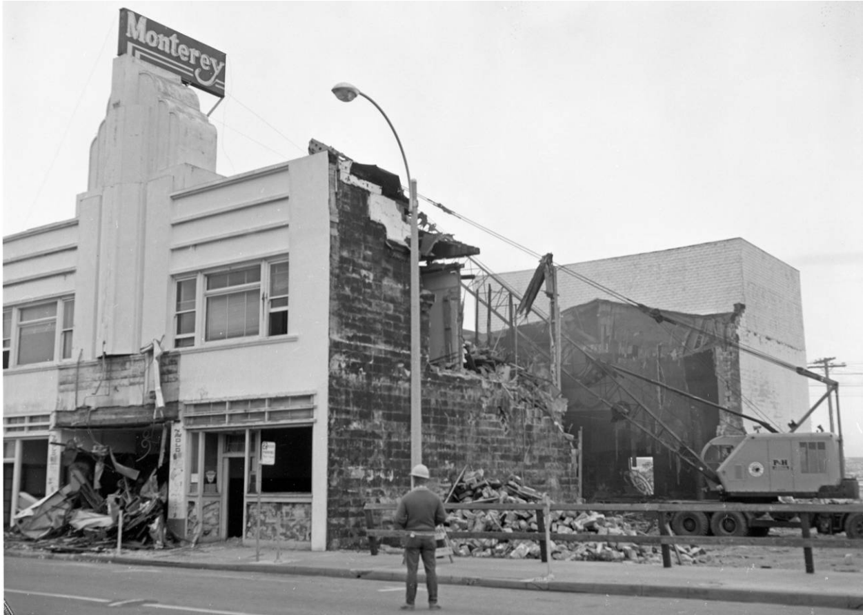
Figure 10-9. Demolition of Monterey Theatre and Kimball shops, February 1, 1967 (William L. Morgan, photographer, courtesy Monterey Public Library, California History Room).
